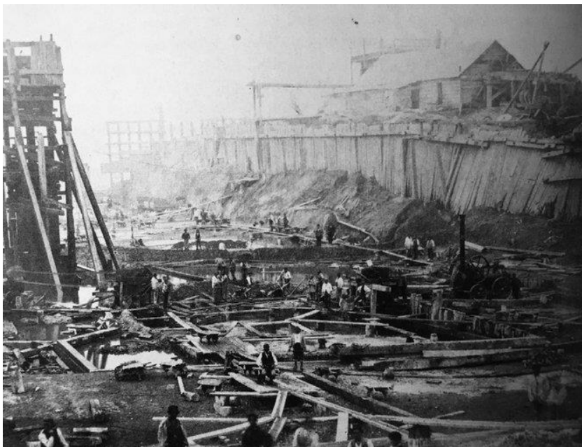
Illus 8: The gigantic scale and nature of the work in 1858 on the old Dock at Grangemouth, most of which was done by hand, can be compared to that at the Albert Dock in Hull in 1867 for which a photographic image survives.
